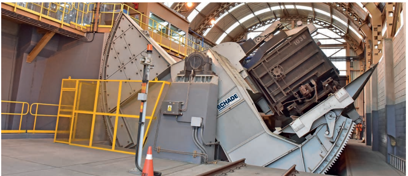
Photo 1: High lift side tipping or 'Pivot Frame' Tippler with shallow foundations (example)
